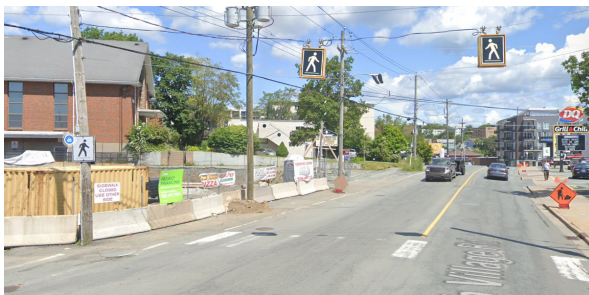
A sidewalk closure due to construction without an alternative path poses a major barrier.
